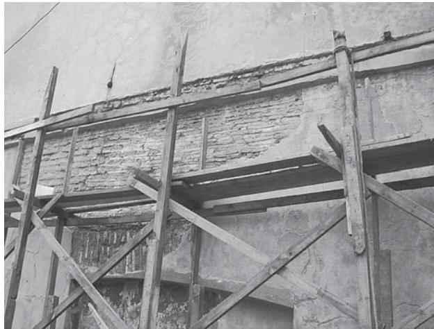
Fig.6 Scaffolding at repair sites is extremely hazardous during earthquakes.
